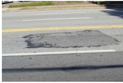
Figure 4 Failed cut on North Avenue (November 2010)
