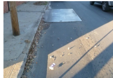
Figure 5 Metal plate on recently paved Grant Street north of Martin Luther King Jr. Drive (January 2011).
