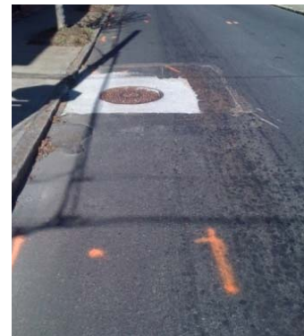
Figure 6 Grant Street north of Martin Luther King Jr. Drive after plate removal (February 2011)
