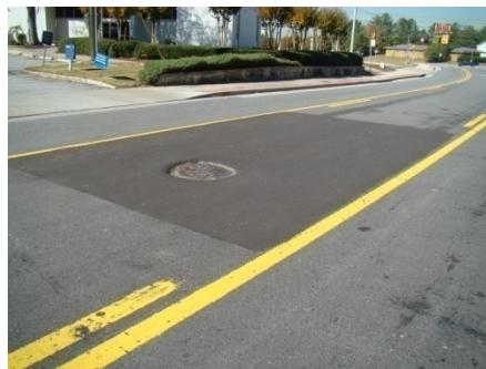
Figure 3 Street cut on Old Gordon Road (November 2010)
