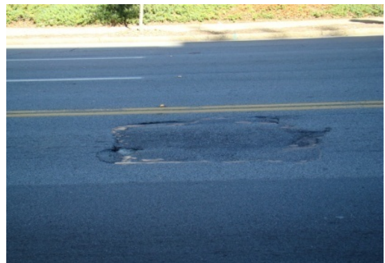
Figure 1 Failed utility street cut located at North Avenue (November 2010)
